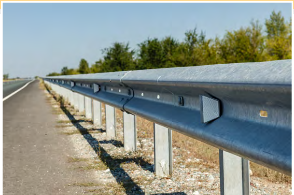
This photo shows a guardrail segment with reflectors, which demonstrates redundancy. The reflectors will help keep vehicles on the road, but if needed the guardrail will prevent vehicles from leaving the road.
